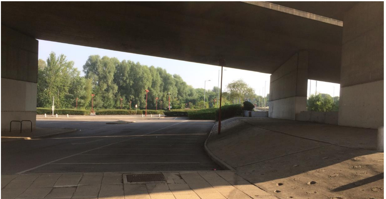
Looking north under the A3290 overpass, including the area of the welfare cabin
